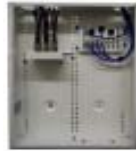
Structured Wiring Panel
