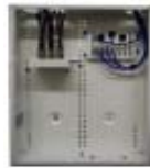
Structured Wiring Panel
