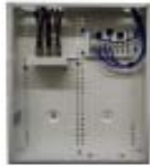
Structured Wiring Panel
